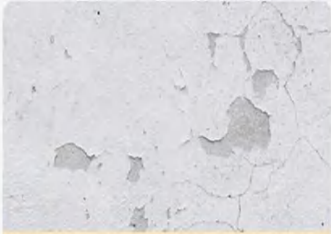
Ash Falling Wall
